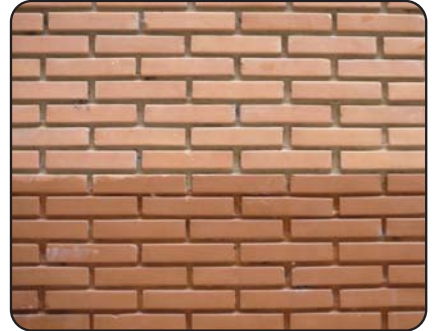
Zahabiya REPECOAT coated on the upper half. The surface looks dry even after rain.
